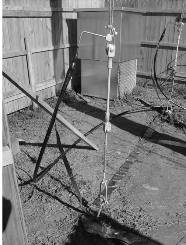
Figure 4 - Kinstar antenna configuration "A" feedpoint showing connection from coaxial matching section to insulated vertical radiator and ground strap from coax outer conductor to ground system. Turnbuckle for tensioning wires and fiberglass insulator are also visible.
